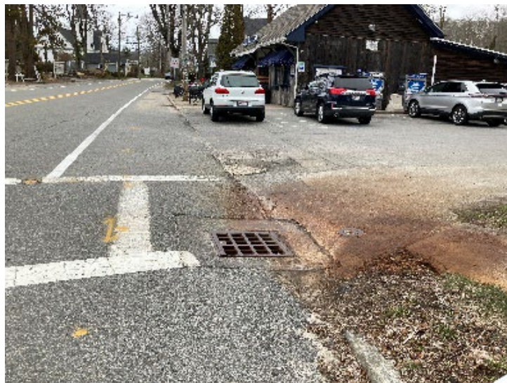
Image 8: Crosswalk at the West Falmouth Market with a Catch Basin in the Path of Travel
