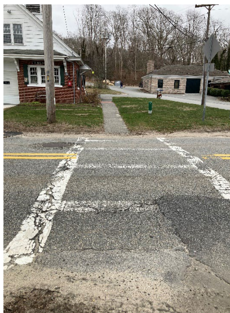
Image 6: Crosswalk with Faded Striping on Route 28A at the Fire Station
